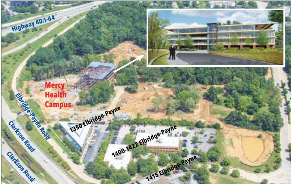
The Mercy Chesterfield Health Campus under construction, with inset sketch of design rendering.
