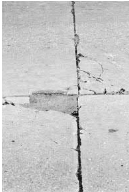
▶ Broken corner pieces. Some joint spalling.
