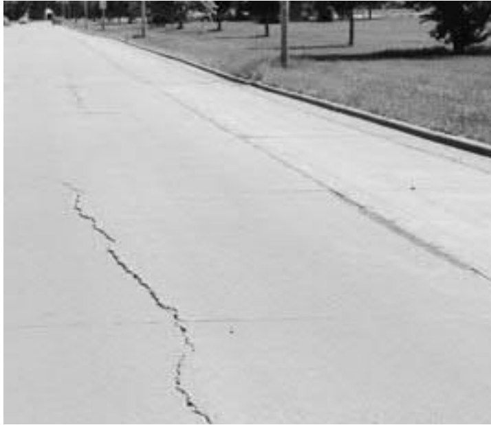
▶ Settlement caused meander crack with faulting.
