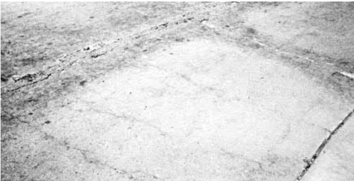
◀ Closely spaced, hairline transverse cracks. Indicates slab is broken and in need of replacement.
