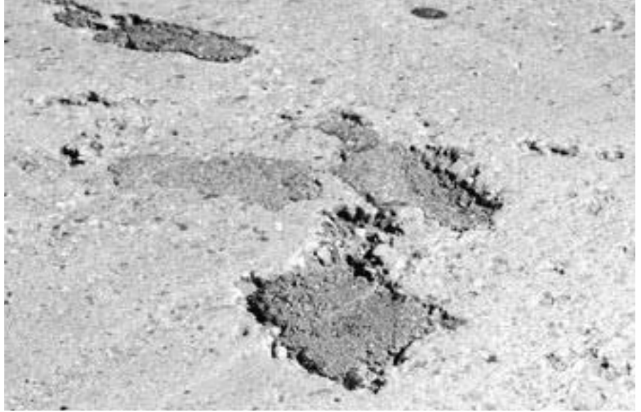
▶ Small surface spalls that have been patched.
