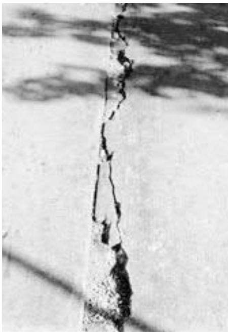
▲ Additional joint cracking, spalling, and broken pavement. Full depth repair is needed.
