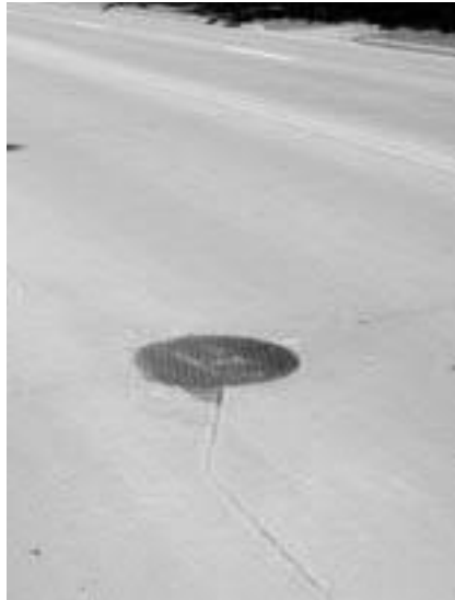
▶ Isolated spall at manhole.
