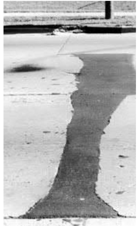
Patching in ▼ fair condition.
