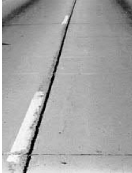
▲ Joint open about 1/2".
