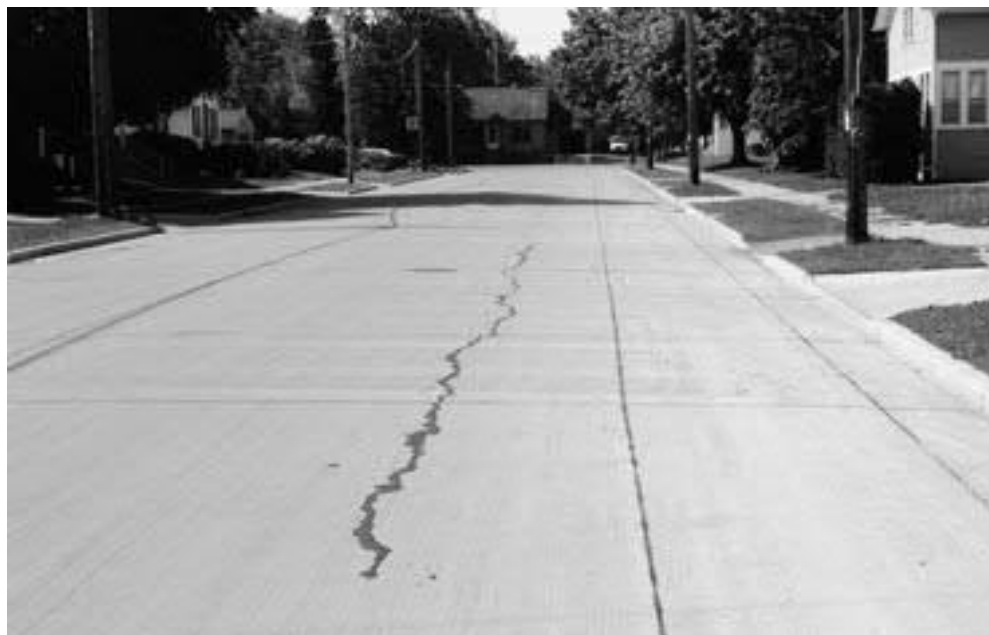
▶ Isolated meander crack, tight and well sealed.
