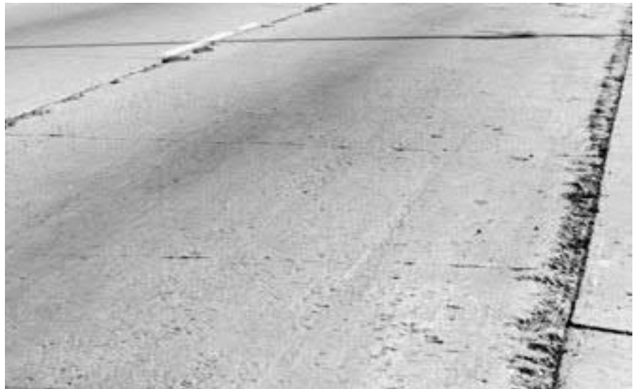
▶ Spalling along longitudinal joints.
