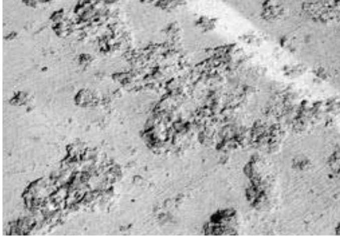
► Moderate surface scaling. Loss of mortar and fines from the surface beginning to expose larger aggregate.
