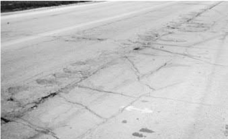
◀ Severe deterioration. Requires extensive reconstruction.
