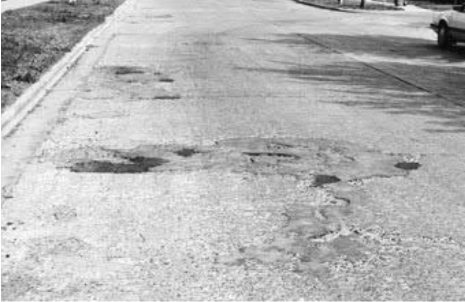
◀ Failed patches. Replace entire portion of lane.
