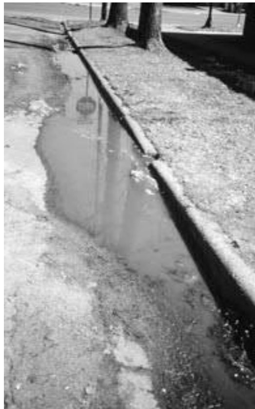
► Flooding. Curb and gutter need reconstruction.
