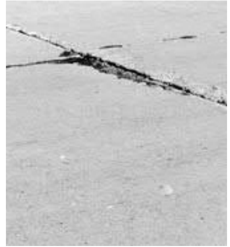
▼ Transverse joint has slight faulting and spalling.
