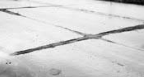
▲ Extensive joint failure. Major rehabilitation or complete replacement needed.
