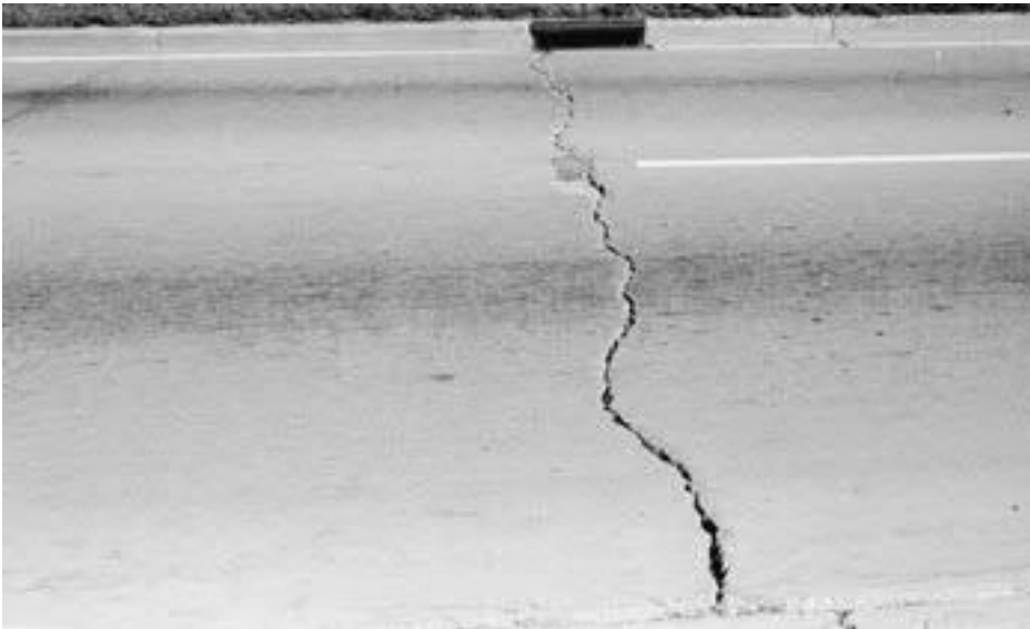
◀ Transverse, open crack.
