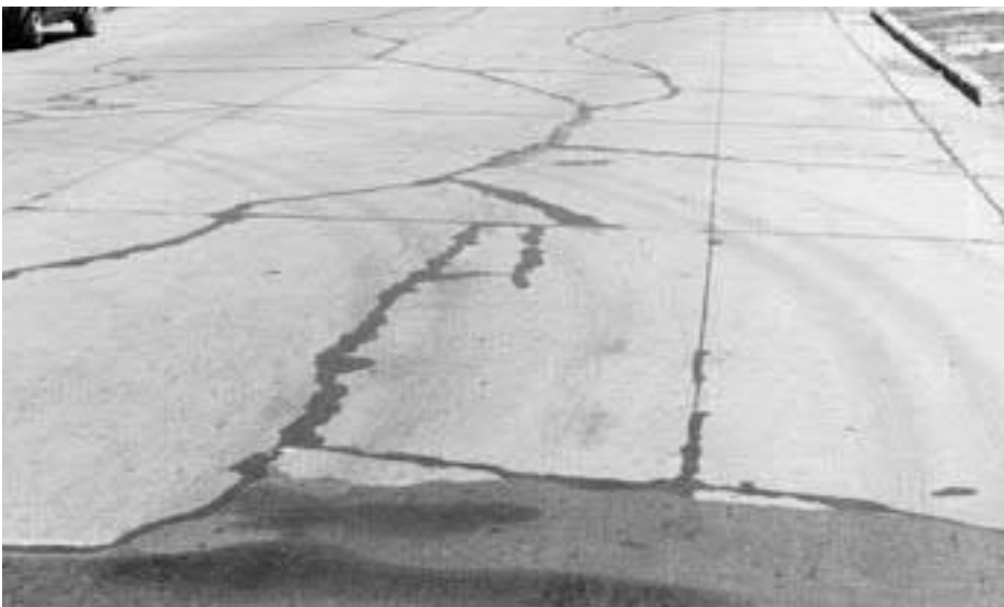
Extensive cracking and patching caused by settlement. Pavement was built on unstable subgrade soils.
