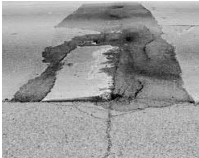
◀ Internal pressure has partially raised slab at the joint. Complete replacement is required.
