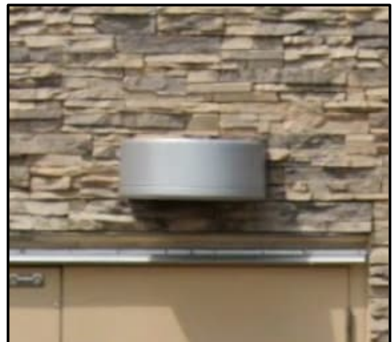
Figure 7: Existing wall mounted lighting
