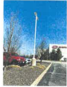
Typical Double Head LED and Lightpole
