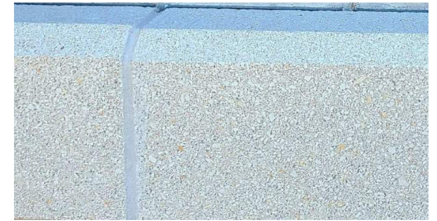
ST1 - CAST STONE CAP CALIBER CAST STONE - MEDIUM GRAY SAME CAST STONE AS ON THE FACTORY BUILDING AND THROUGHOUT THE CENTER
