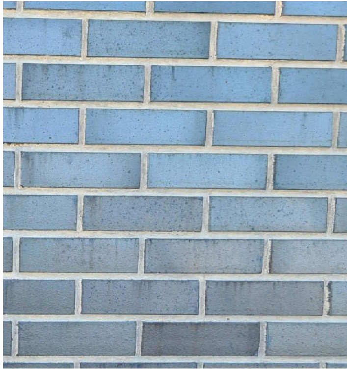
BR1 - THIN BRICK VENEER GLEN GREY BRICK SAME BRICK AS ON THE FACTORY BUILDING
