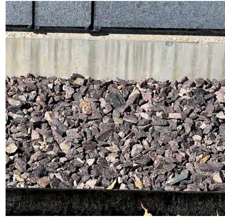
GRAVEL MAINTENANCE STRIP (SEE LANDSCAPE) 3/4" - 1" CLEAN ANGULAR TRAP ROCK 5" X 1/4" STAKED STEEL EDGING, BLACK POWDERCOAT
