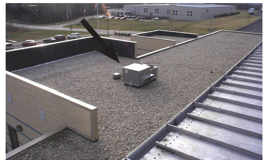
(ii.) The parapet wall and its location on the roof help hide the condensing unit from street.
