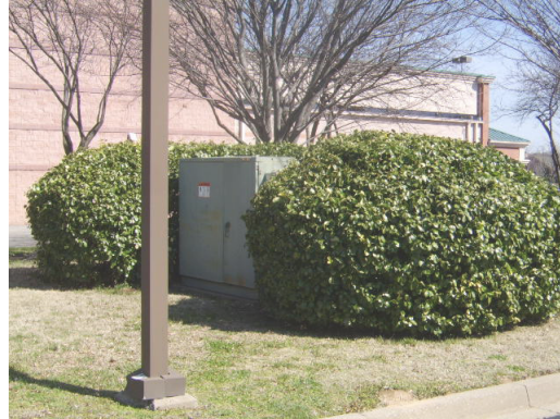
Utility cabinet is screened on three sides by shrubs
