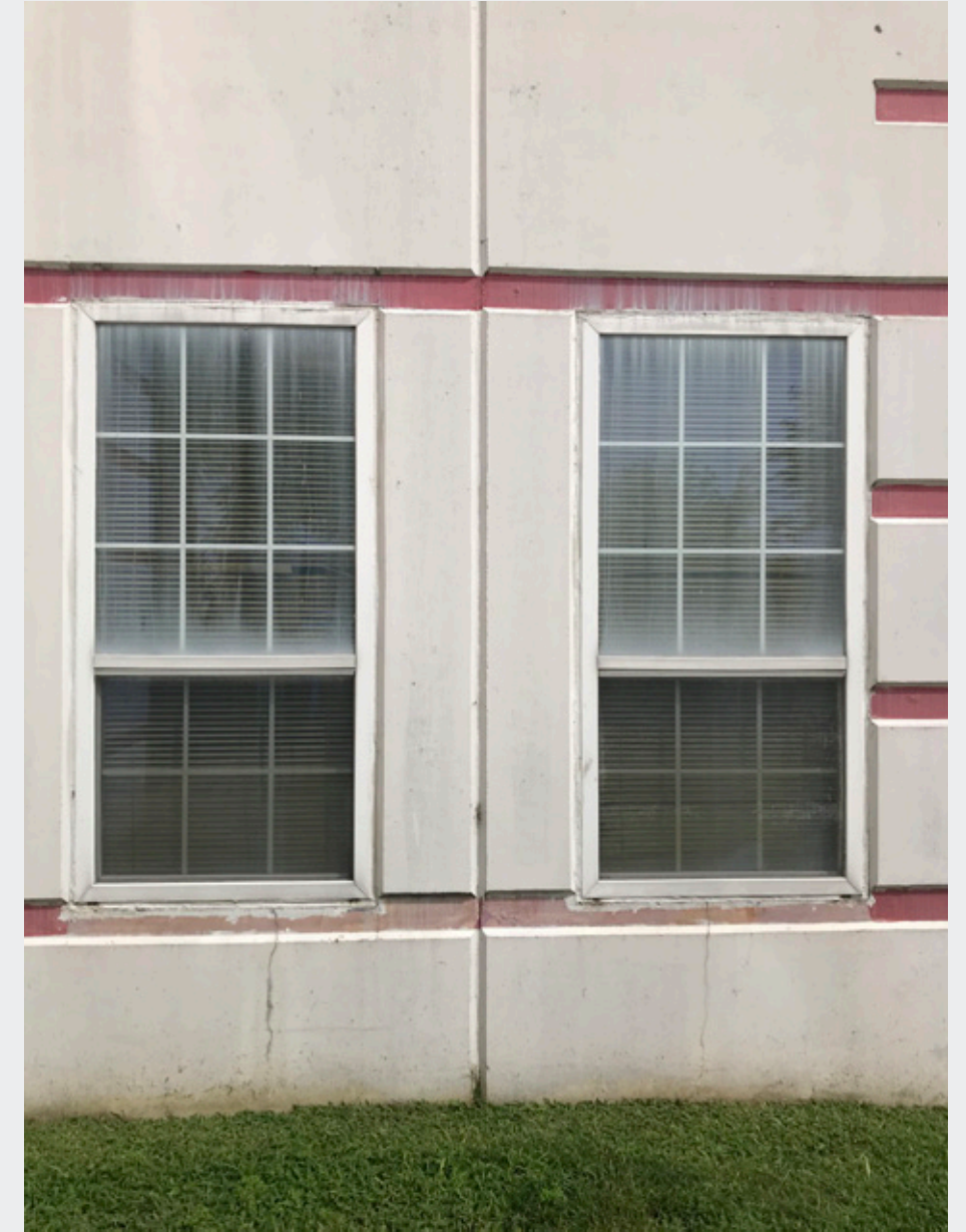
Existing Windows Note: we will NOT be replacing with double hung units. We will NOT be using divided lites. As proposed will be single pane of glass (IGU) with head, jambs and sill
