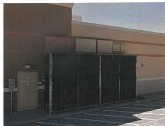
EXISTING SCREENING SYSTEM FOR ELECTRICAL SWITCHGEAR
