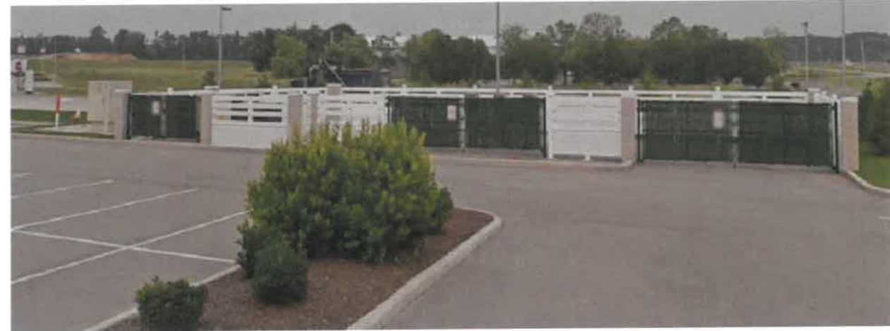
EXISTING SCREENING SYSTEM FOR SANITARY PUMP STATION
