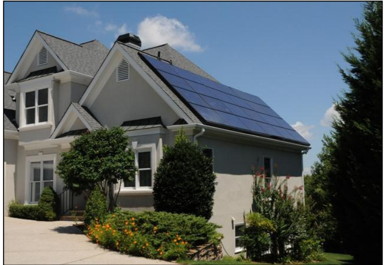
Image 1: A residential PV installation in Johns Creek, GA.
