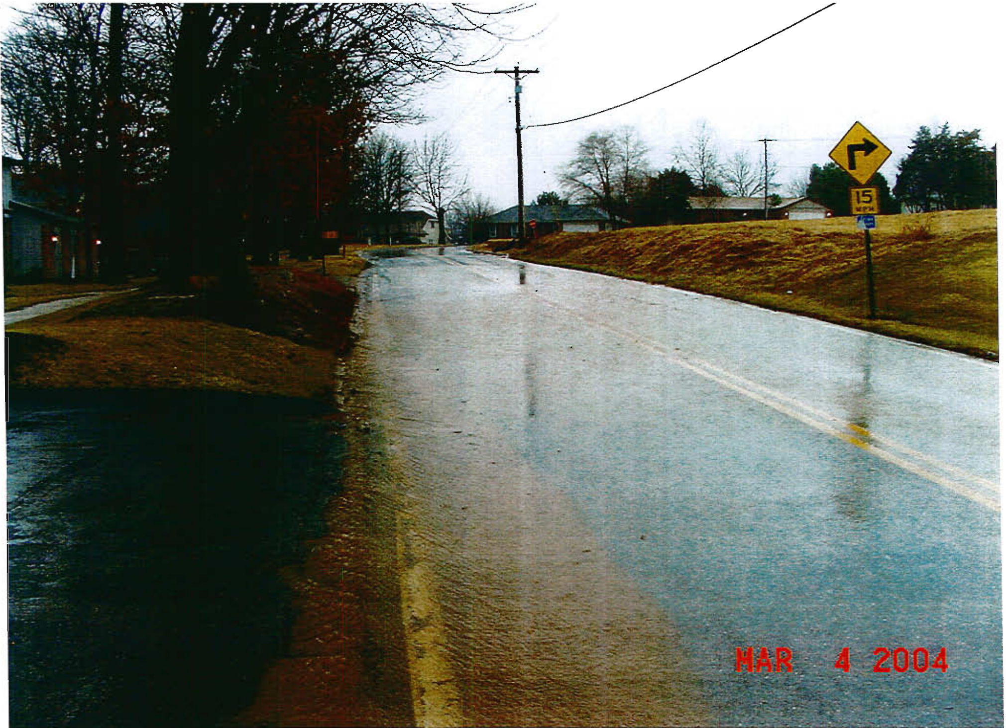
Old Baxter - Looking south showing water in east gutter line.JPG
