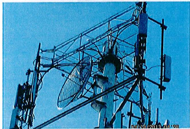
PHOTO OF EXISTING ANTENNAS
