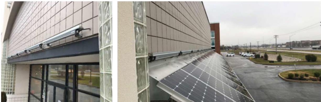
Figure 5: Photos of permanently mounted light fixtures
