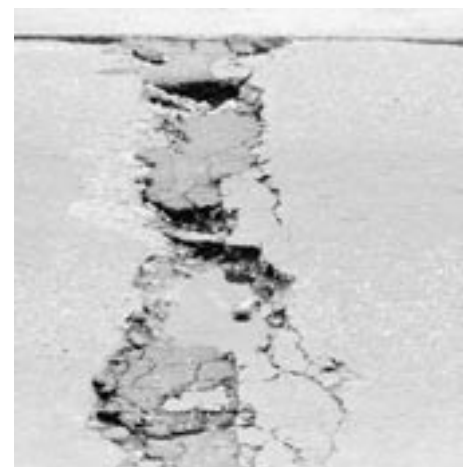
▲ Potholes caused by severe joint deterioration. Need repair.
