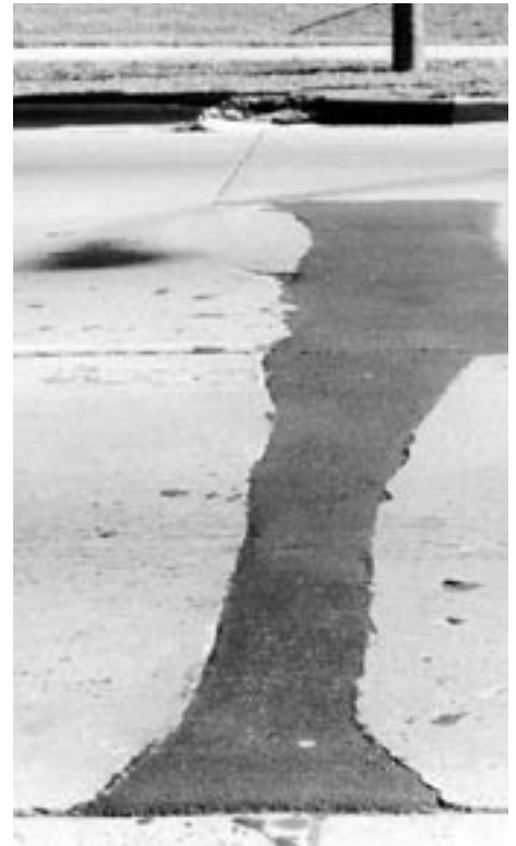
Patching in ▼ fair condition.
