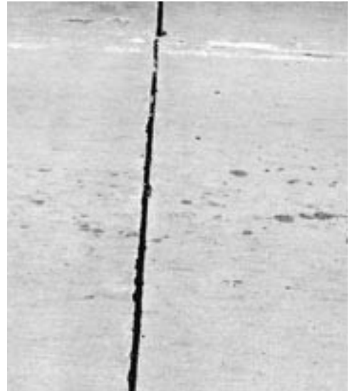
▲ Partial loss of joint sealant.
