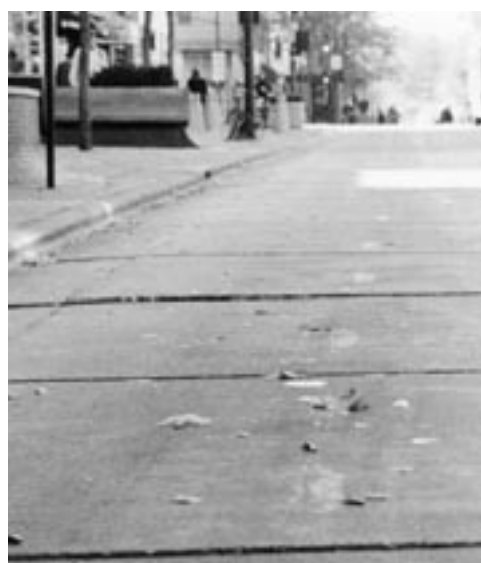
▲ Minor faulting of transverse joints. Aggravated by heavy traffic. Surface grinding will improve ride.
