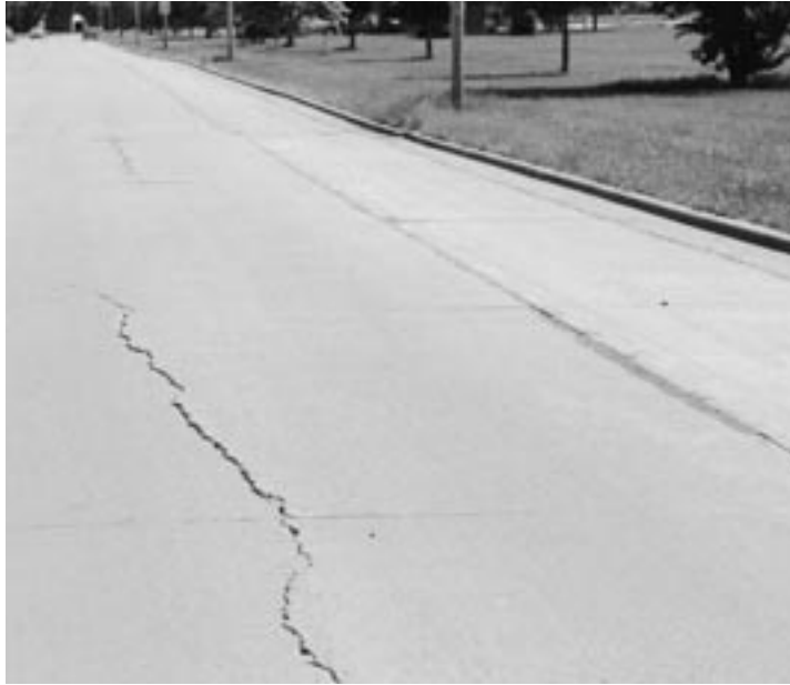
► Settlement caused meander crack with faulting.
