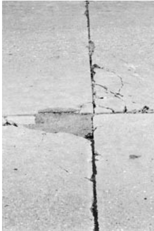
▶ Broken corner pieces. Some joint spalling.
