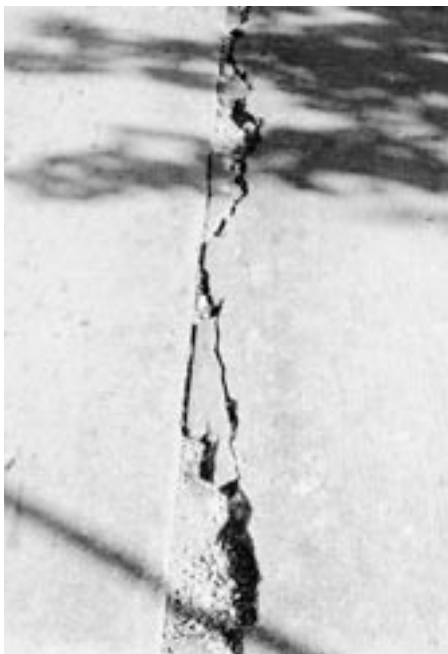
▲ Additional joint cracking, spalling, and broken pavement. Full depth repair is needed.
