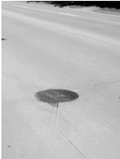
▶ Isolated spall at manhole.
