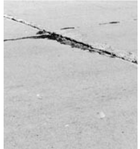
▼ Transverse joint has slight faulting and spalling.
