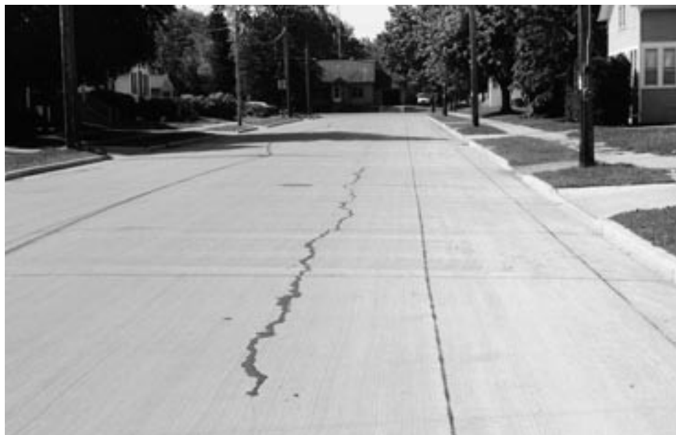
▶ Isolated meander crack, tight and well sealed.
