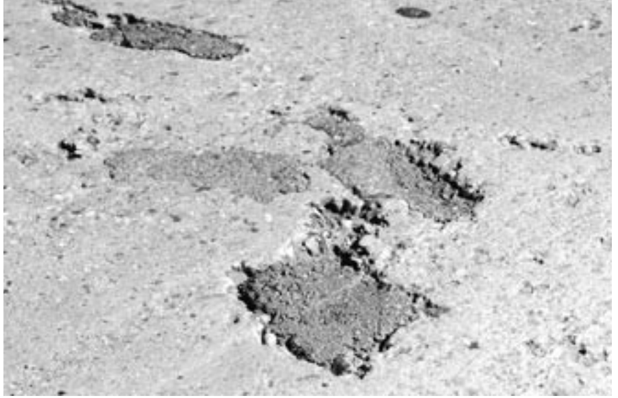
▶ Small surface spalls that have been patched.
