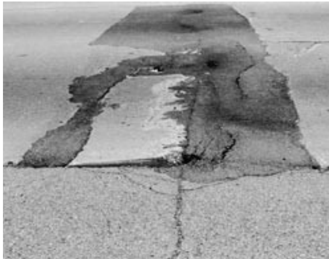
◀ Internal pressure has partially raised slab at the joint. Complete replacement is required.
