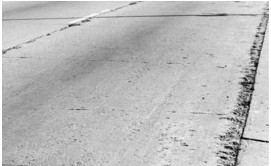
▶ Spalling along longitudinal joints.
