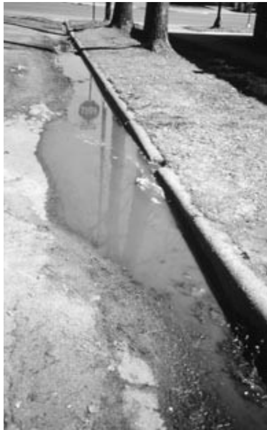
► Flooding. Curb and gutter need reconstruction.
