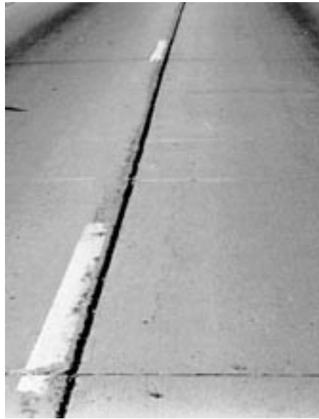
▲ Joint open about 1/2".
