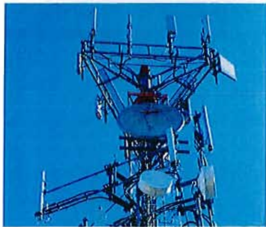
PHOTO OF EXISTING ANTENNAS
