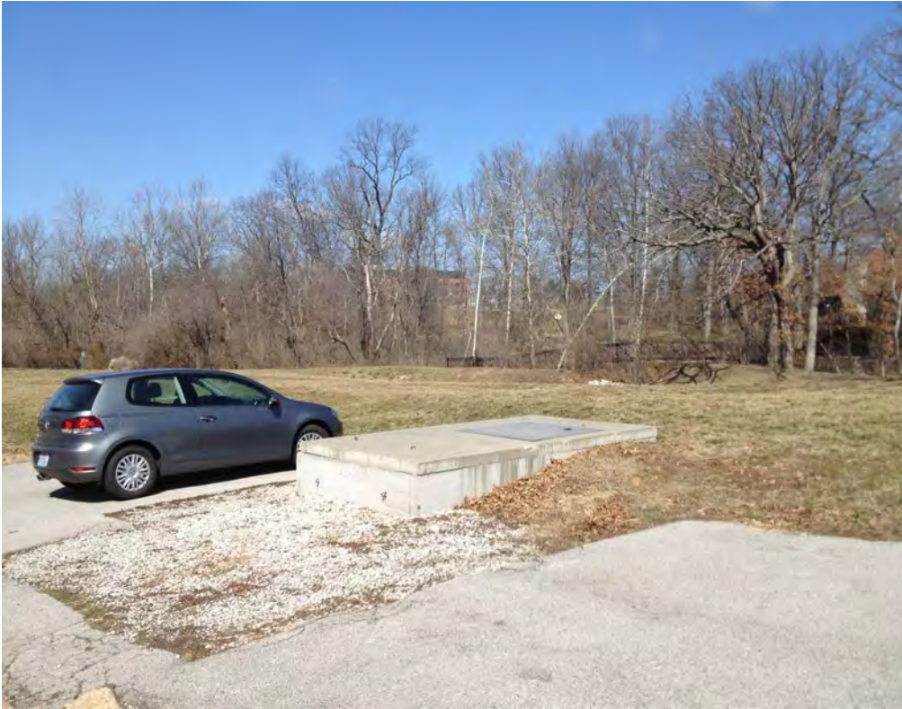
View of the existing water valve box that serves the existing condos to the East
