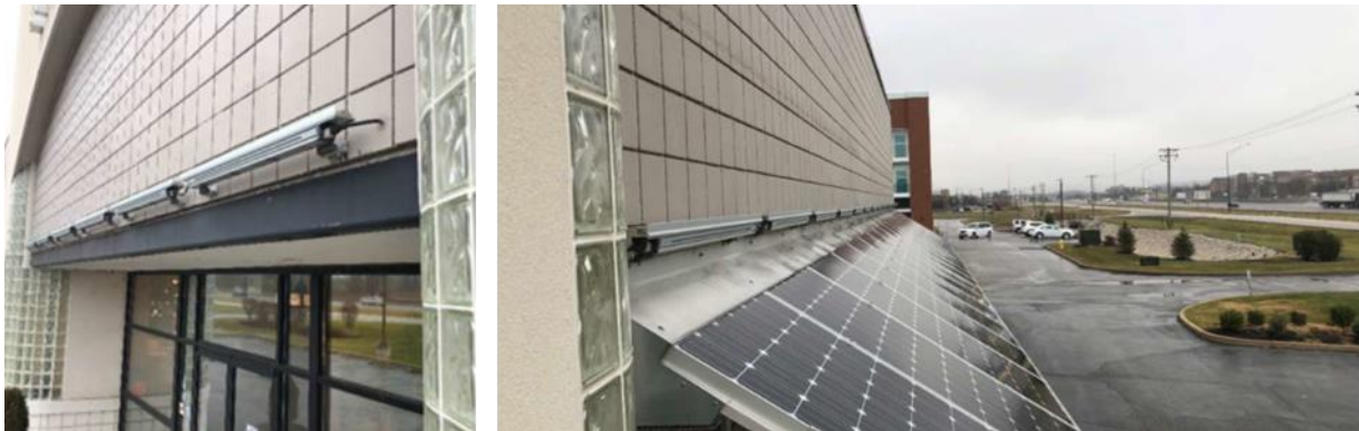
Figure 5: Photos of permanently mounted light fixtures
