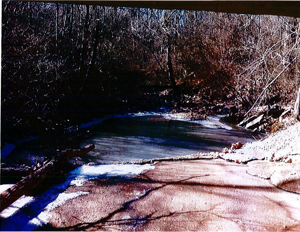
PHOTO E: VIEW DOWNSTREAM – INVERT TOO HIGH
