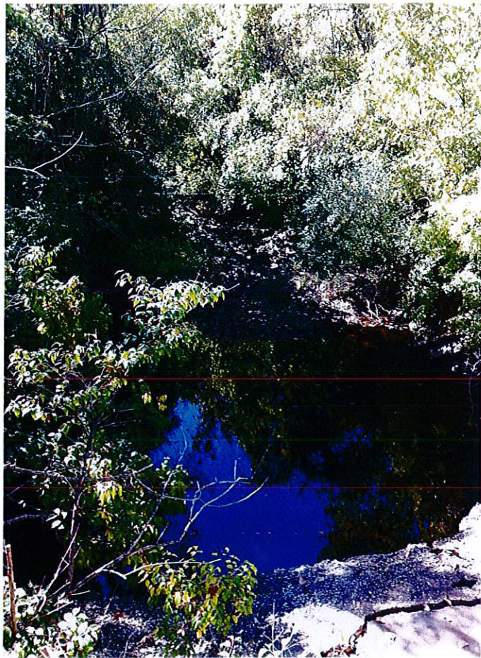
PHOTO G: DOWNSTREAM SCOUR HOLE
