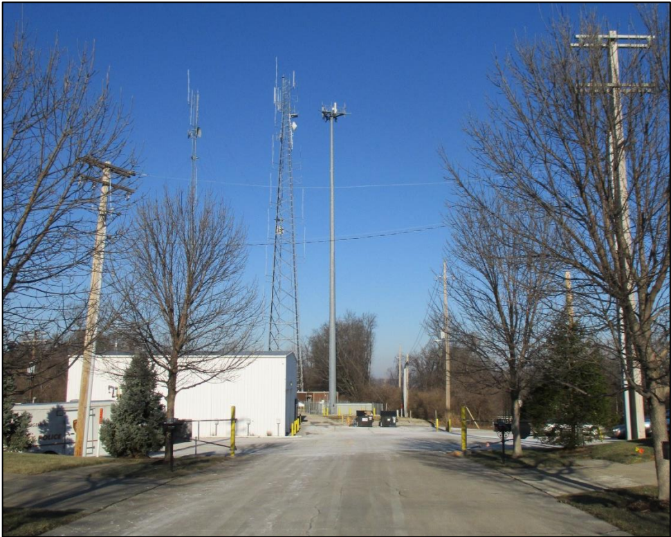
Figure 3: Closer Photo of Towers- Monopole to the Right is the Tower in Question
