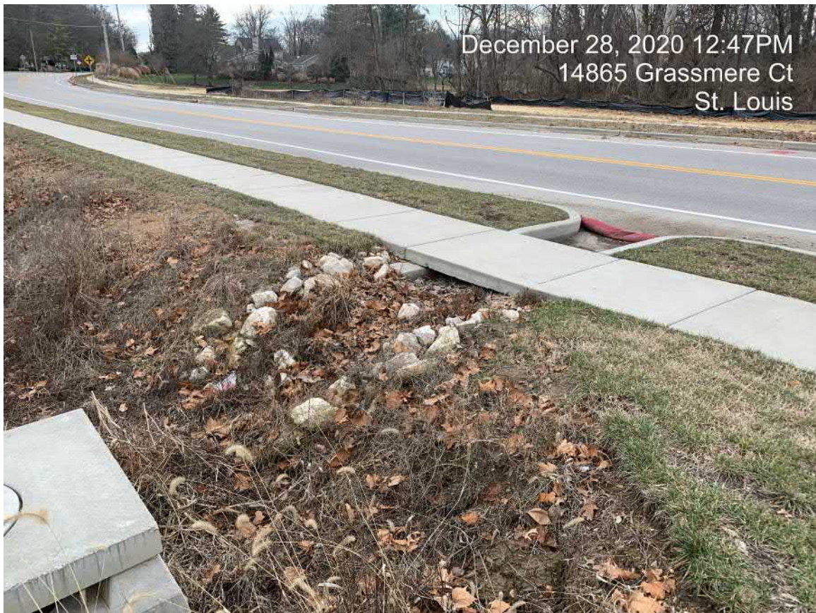
Scupper on East Side of Schoettler Road south of the Schoettler Road Bridge.
