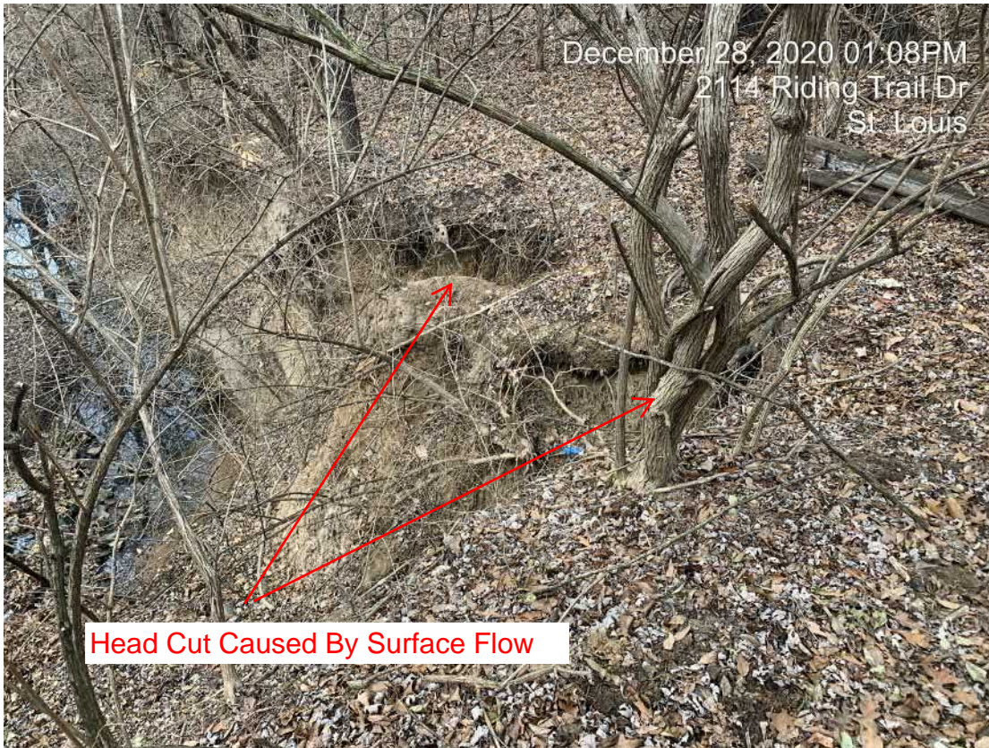
Eroded Banks of Existing Drainage way.
