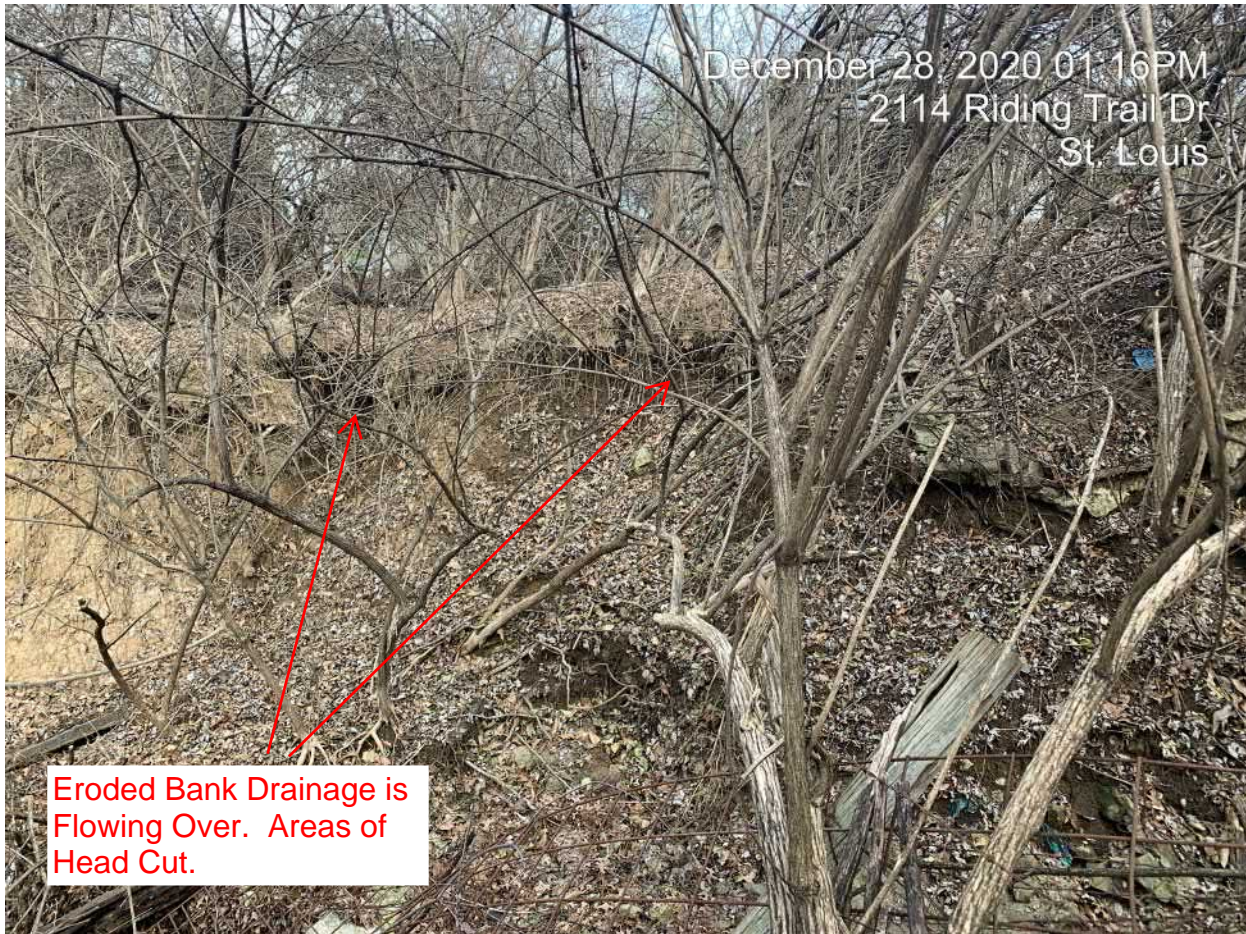
Unstable Bank of Existing Drainage Way. Looking From Flow Line of Drainage Way.
