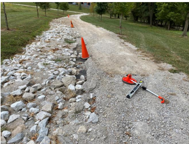
Figure 4: West end of north leg of South Trail loop. Geofabric exposed after continued erosion.
