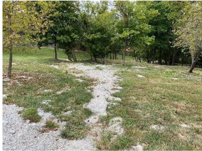
Figure 5 – Washout at the northwest corner of the Southern Trail
