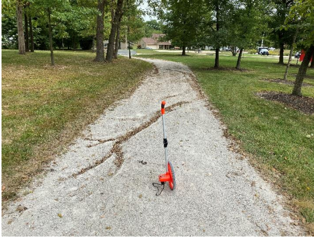
Figure 11 – Northeast corner of the North Trail, facing east, erosion occurring from stormwater draining from the north (left in photo).
